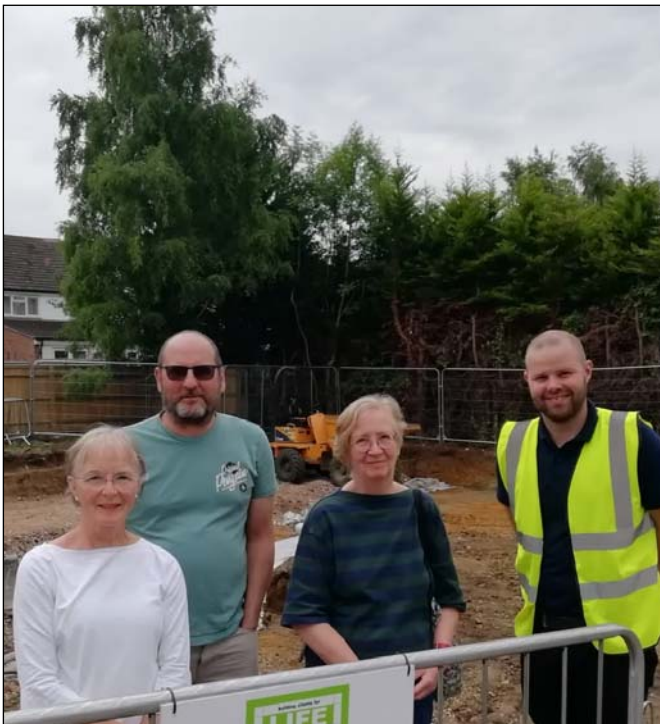
Site Manager Kevin McGowan (right) with some of the OCLT directors on site
